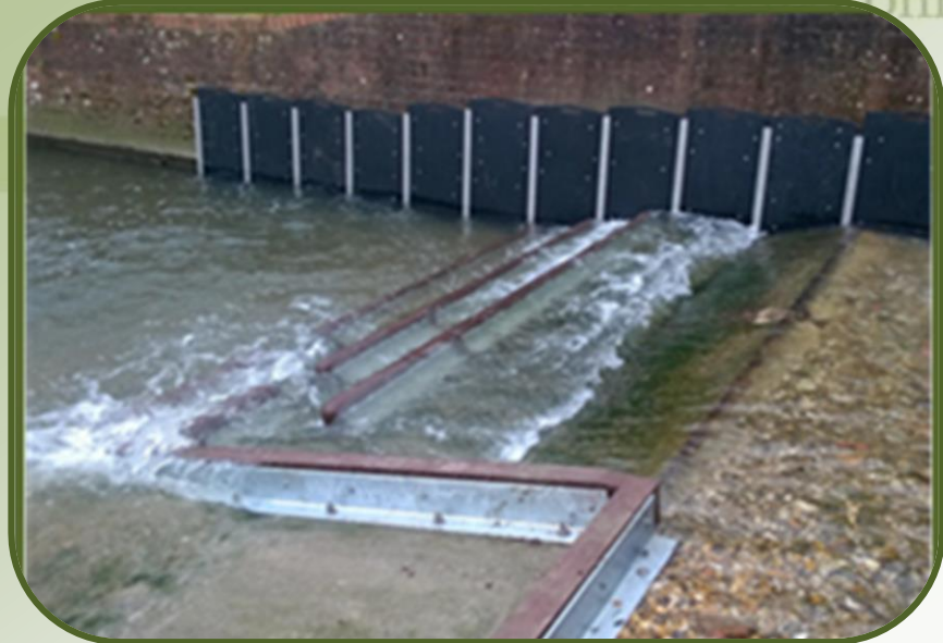
One of the recently installed baffle fish passes on an EA gauging weir
